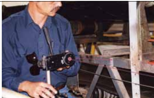
Figure 16.12 The beam of light from a laser transit provides an unobstructed and repeatable reference for the alignment of the conveyor-structure components.
