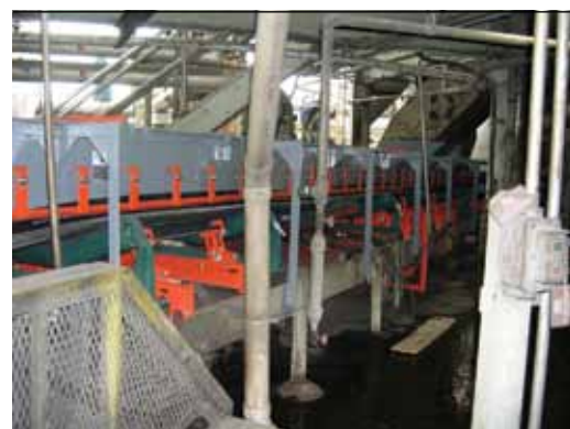
Figure 8.6 A conveyor can have its service-friendly capabilities canceled out by the placement of utility piping and conduits and other components.
